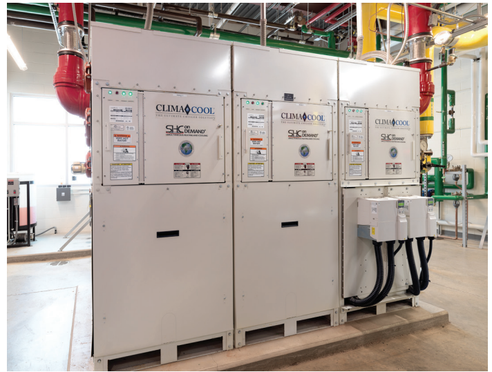
ClimaCool modular water-to-water heat pump installed in the Canyon Creek Elementary School.
