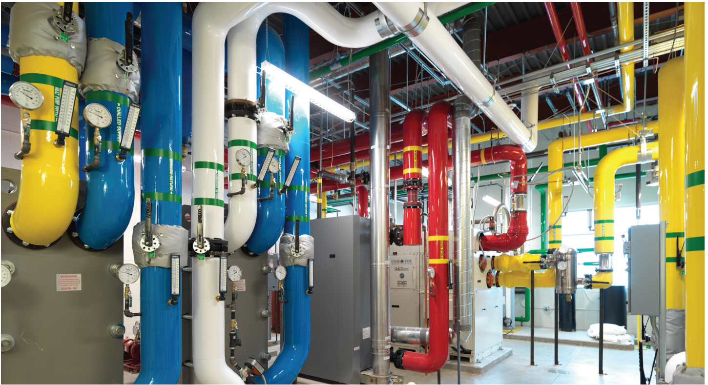
The mechanical room of the Odyssey Elementary school contains some of the equipment comprising the innovative system with indirect evaporative cooling, daylight harvesting, solar panels and a geexchange heating and cooling. The ClimaCool geothermal heat pump is visible in the center.
